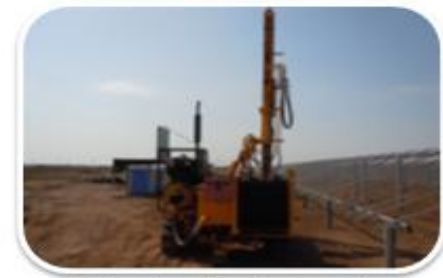
Grid tied solar photovoltaic structural Engineering, Procurement & Commissioning (EPC)
