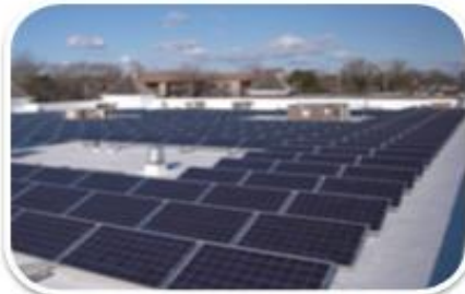
Off-Grid Solar (Home Made) solar photovoltaic (PV) electricity system integration
