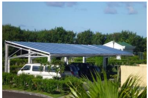
SOLAR CAR PARK
